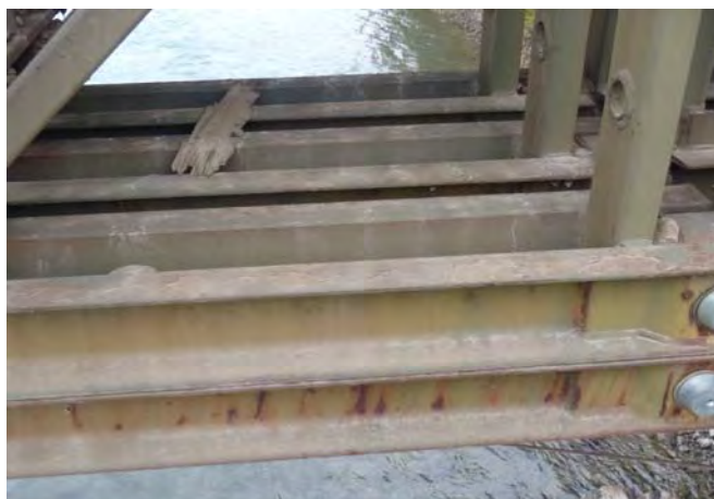
Figure 1-18: Typical peeling paint and minor surface corrosion of panel.
