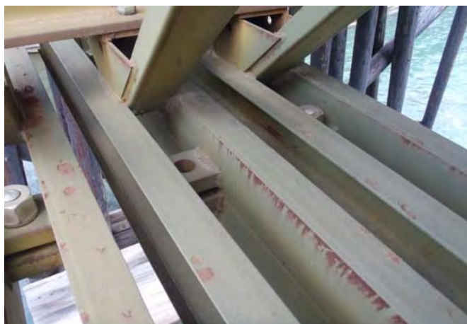
Figure 1-17: Typical missing reinforcing connection bolt in span 2 downstream panel 9.
