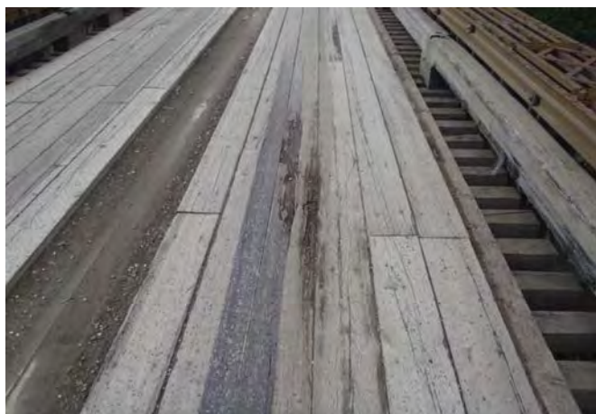
Figure 1-11: Pocket of rot in running strip.
