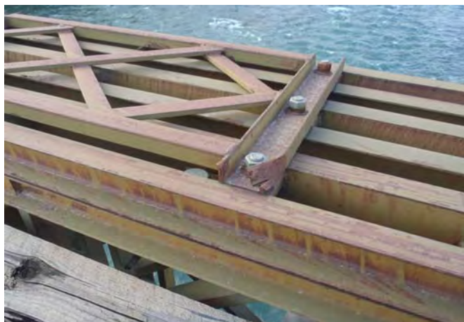
Figure 1-13: Typical impact damage to bracing frame.
