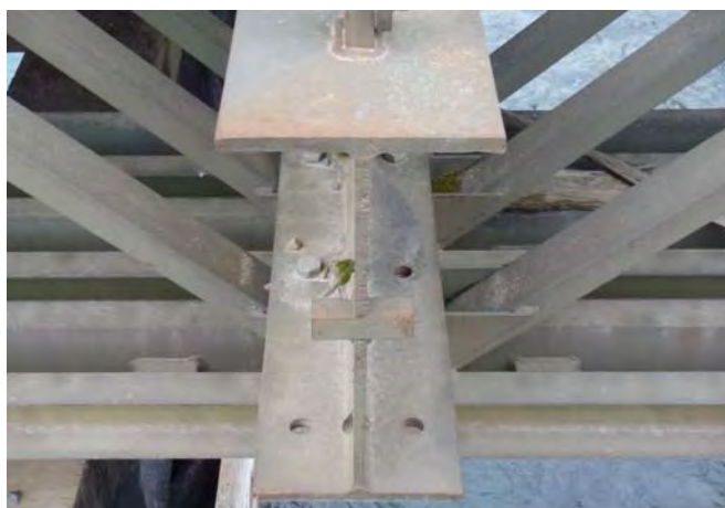
Figure 1-16: Typical missing transom bolts, span 3 panel 1 shown.
