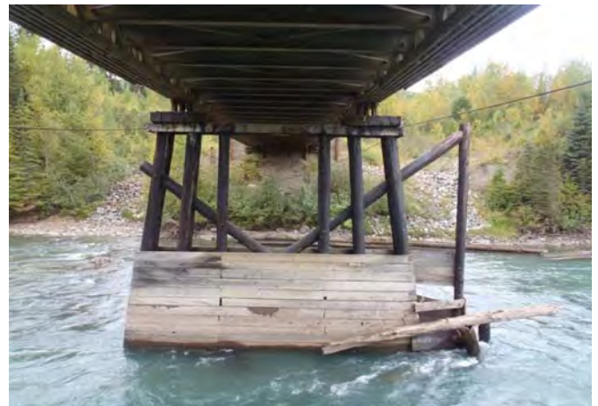
Figure 1-28: Pier 2 Wells end face, log jam and missing sheathing panels.
