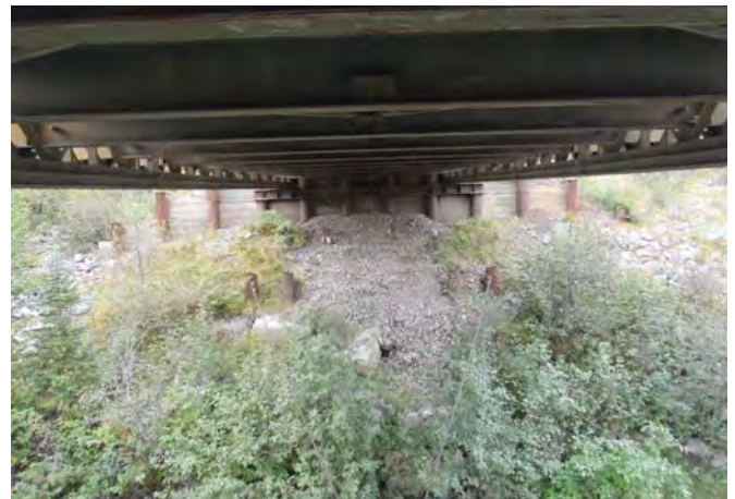
Figure 1-22: Likely end abutment, note over turned lock blocks.
