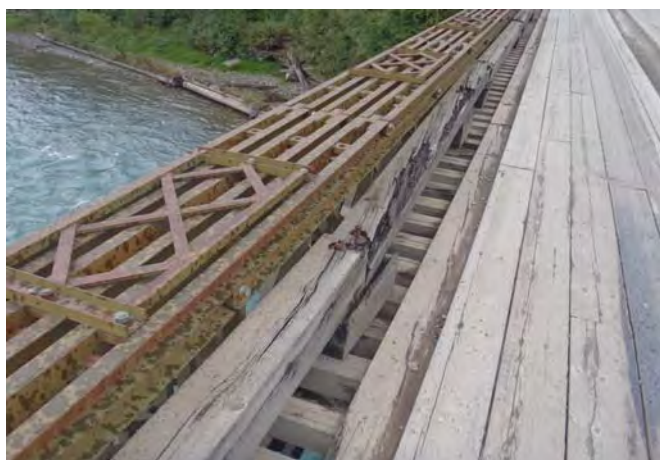
Figure 1-9: Pocket of rot on curb rail, upstream shown.
