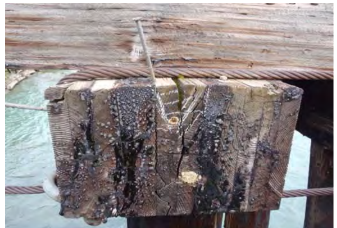
Figure 1-30: Typical end check in cap, Pier 2 likely end downstream shown.
