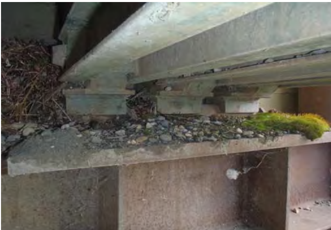
Figure 1-23: Typical abutment bearing condition debris accumulation Likely end upstream shown.
