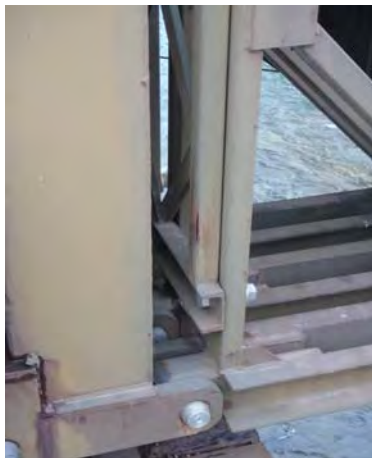
Figure 1-21: Span 3 pier 2 upstream panel, crack in end post.
