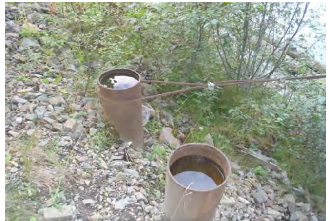
Figure 1-24: Pier 2 Likely end dead man piles, full of water.
