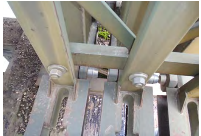
Figure 1-20: Typical protruding panel pin due to missing safety clip.
