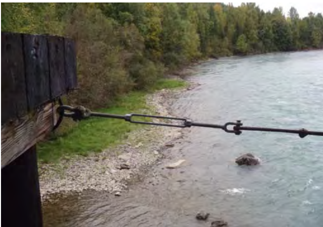
Figure 1-27: Typical loose cable sway brace, Pier 1 downstream shown.
