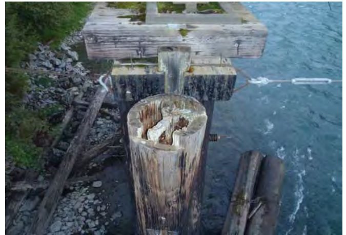
Figure 1-26: Pier 1 dolphin pile, heartwood rot.
