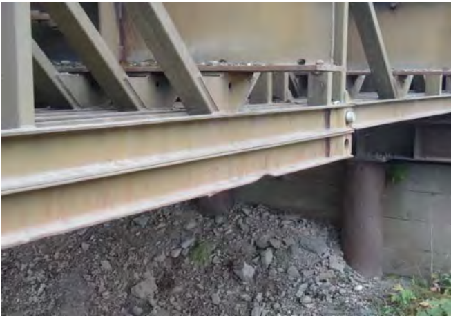
Figure 1-19: Minor damage to bottom chord reinforcing in span 3 panel 9 upstream.
